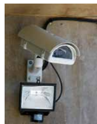
Exterior Security Lighting
